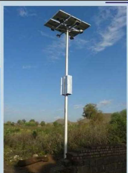
Solar High Mast Light
