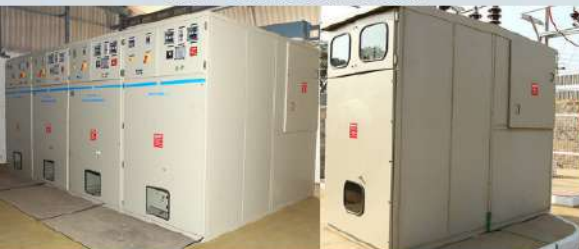
HV VCB Panels
